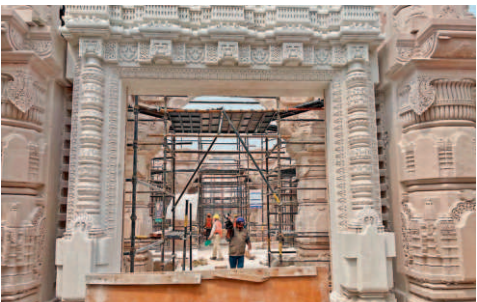
The work to place beams above ground floor pillars at the Shri Ram Jambhoomi Mandir has started. Some beams have already been placed, tweeted Shri Ram Jambhoomi Teerth Kshetra Thursday.
